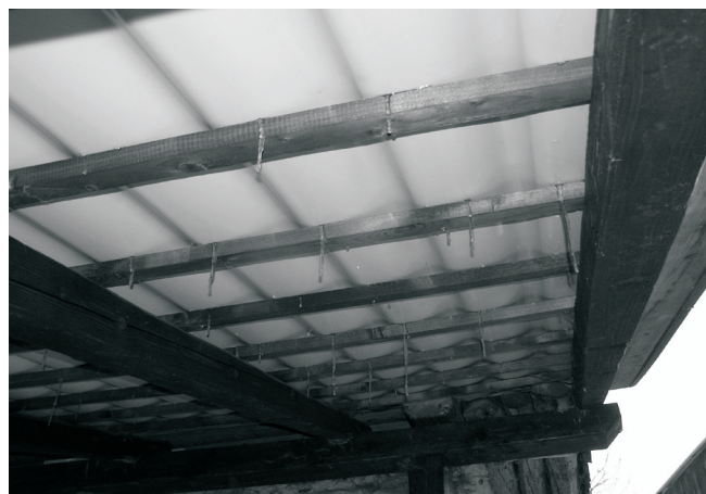
Fig. 2.2 Leaking of screw joints in the winter.
