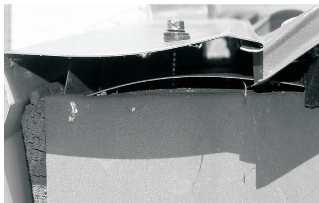
Fig. 2.4 Incorrectly mounted anchorage screw with an uncompressed sealing washer.
