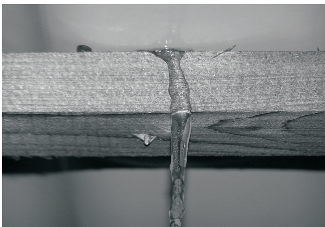
Fig. 2.1 Detail of leaking water through the screw joint of the sheet roofing imitating a roof tile in the winter.
