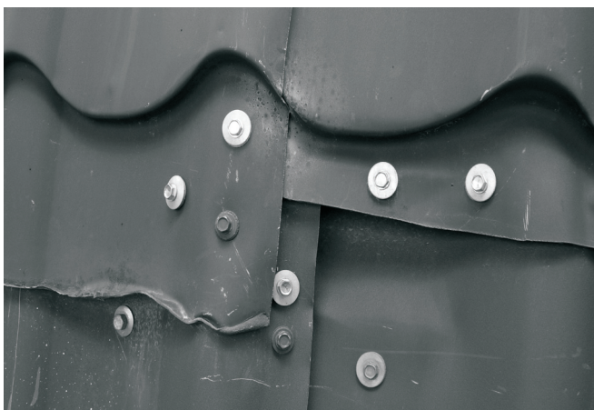
Fig. 2.6 The anchoring of a sheet with a lot of screws and unprofessional cutting.
